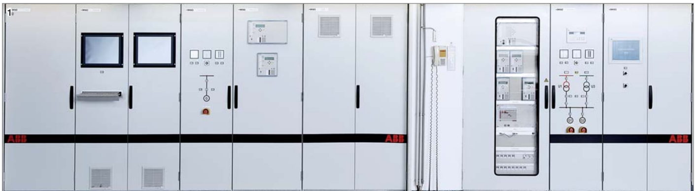
1 and 2 Marchtrenk hydropower plant (Austria) - Unit control board and an AC800M control cubicle (interior) 3 Kops II (Austria) - Unit control board screenshot
